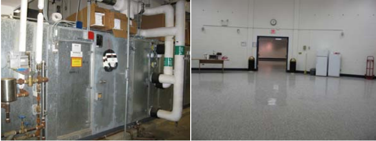
Photo 10: 1 st Floor mechanical room, view of air conditioning units
