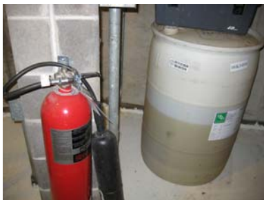
Photo 1: Room 206A, view of chemicals and fire extinguisher
