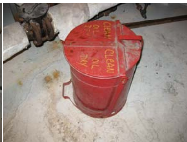
Photo 2: Room 206A, view of oily rag drum
