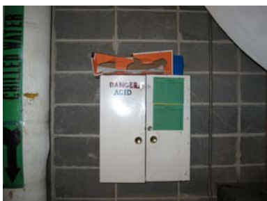
Photo 7: Room 206A, view of acid cabinet
