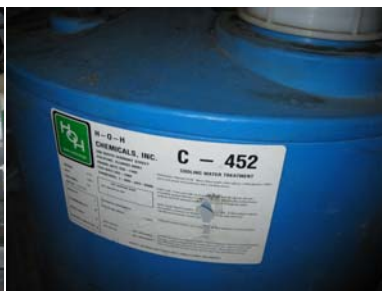
Photo 5: Room 206A, view of hazardous chemical drum
