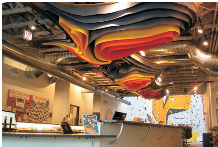
FIGURE 7. This is an interesting soundproofing installation at First Ascent, Chicago. The installation is not only aesthetically pleasing, but it also serves a functional purpose: to provide a barrier for vibration and noise from the heating and cooling ducts. (Courtesy, Fabric Images, Inc., Elgin, IL)
